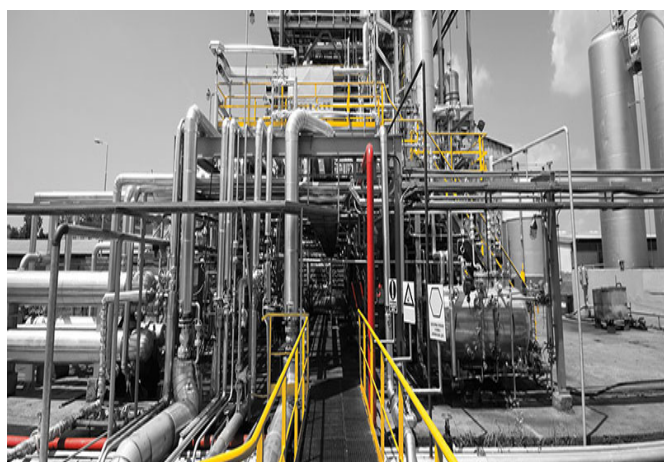
Gas & Oil Factories, Hot Pipe & Floor Area
